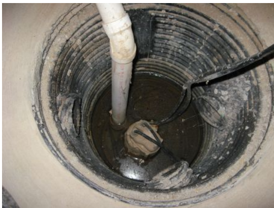
Figure 6.15: A sump crock.
